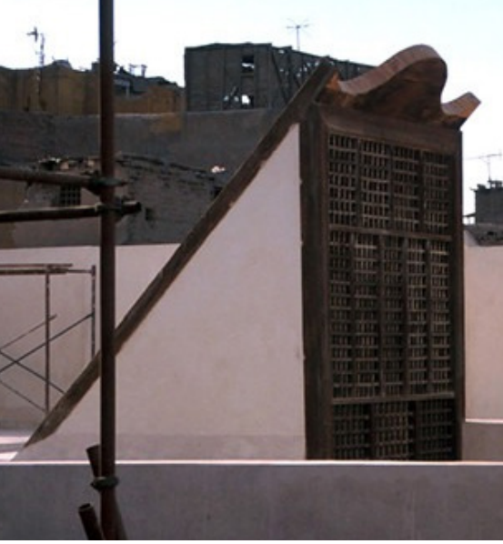
Malqaf Capturing fresh air for a natural supply
